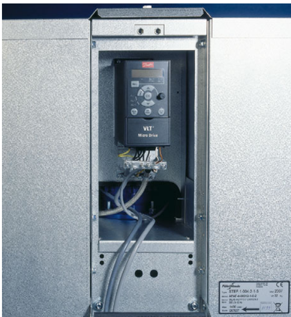
Frequency converter mounted into roof fan.
